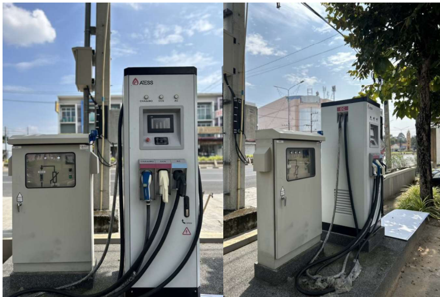
5. EV stations (Ubon Ratchathani Rajabhat University, Thailand)
