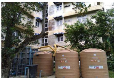
Tanks for recycled water
