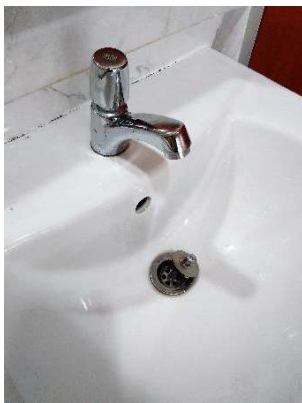
Efficient tap found in many buildings
