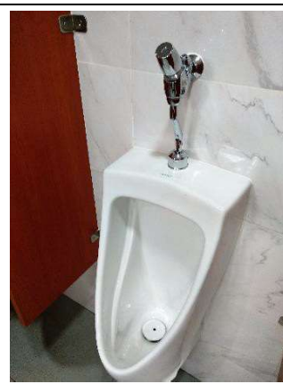
Efficient urinal flush found in most buildings
