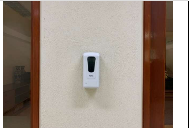
Install an alcohol-gel hand-washing machine before entering the meeting room
